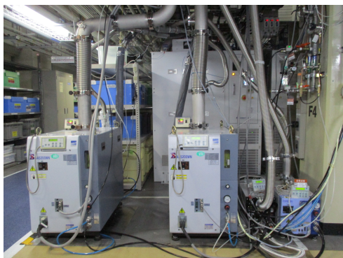
PFC除害設備
