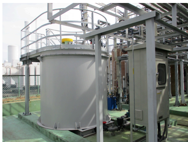
Acid treatment equipment
