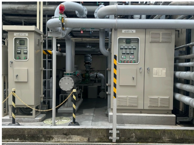
Room temperature cooling water pump panel after update
