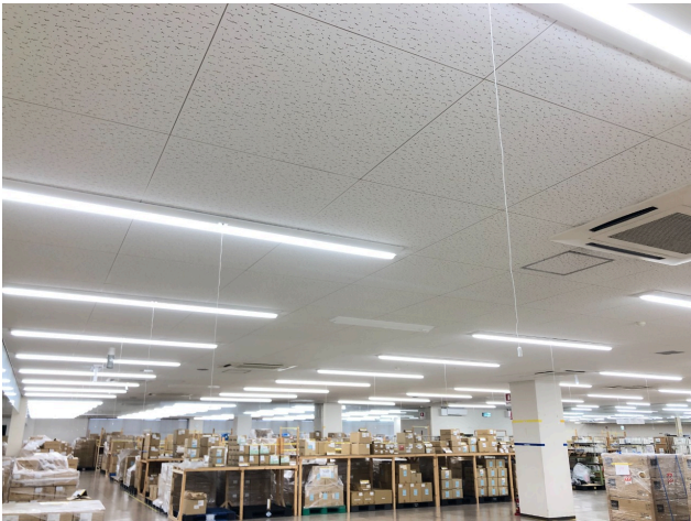
LED lighting fixtures
