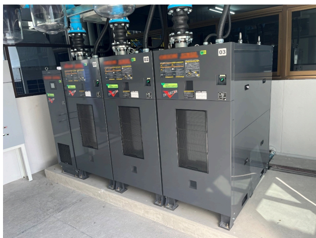
Central vacuum pump
