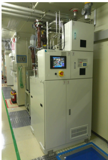
PFCs and other gas abatement equipment
