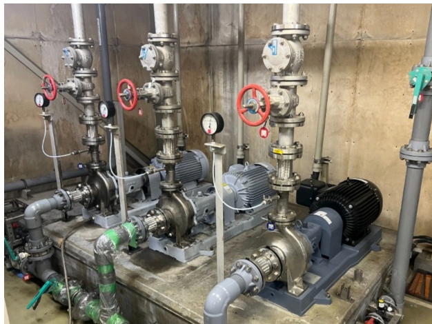
RO high pressure pump after update
