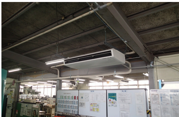
Air-cooled air conditioner
